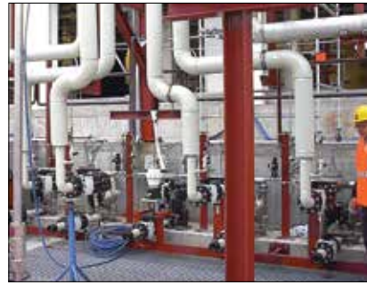
2" stainless steel diaphragm pumps assembled with PVDF pulsation dampeners used to download hydrofluoric acid
