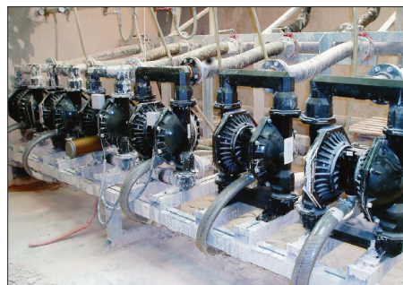
3" diaphragm pumps mounted on a skid to transfer clay in a ceramic manufacture
