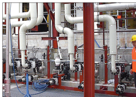
2" stainless steel diaphragm pumps assembled with PVDF pulsation dampeners used to download hydrofluoric acid
