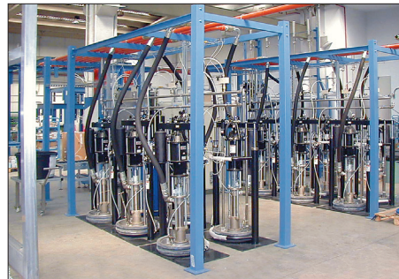
Large extrusion piston pumps, 13:1 ratio, installed on an offset ink formulation system process
