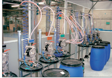
1/2" diaphragm pumps installed in a coloring process
